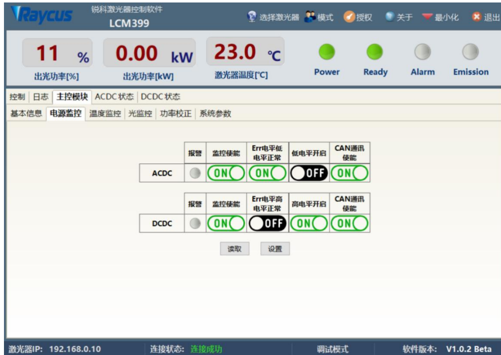
Figure 17 Alarm information interface of main control module
